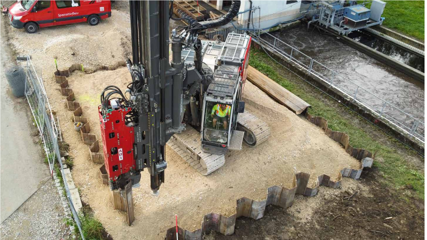
Photos: ABI MOBILRAM TM 14/17 SL while working at the job site in Inzigkofen-Vilsingen (above) Loading the machine for the transport to the next job site (below)
