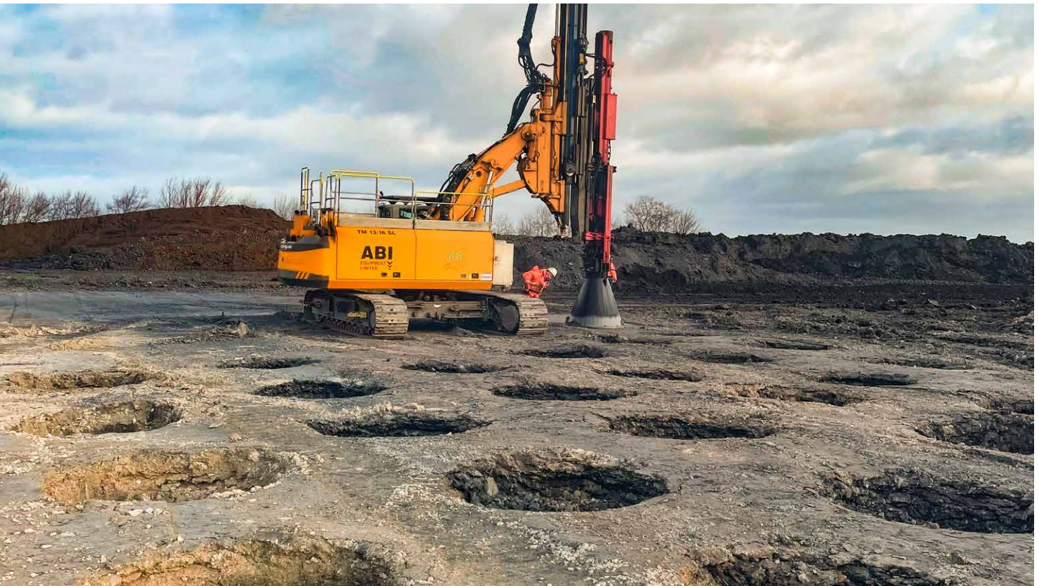
Photo: ABI MOBILRAM TM 13/16 SL with DELMAG diesel pile hammer D19-52 and compaction foot
