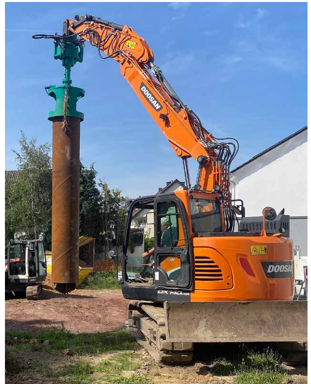
Photo: cased drilling with ABI excavator mounted auger drive BA 2200 and casing twister
