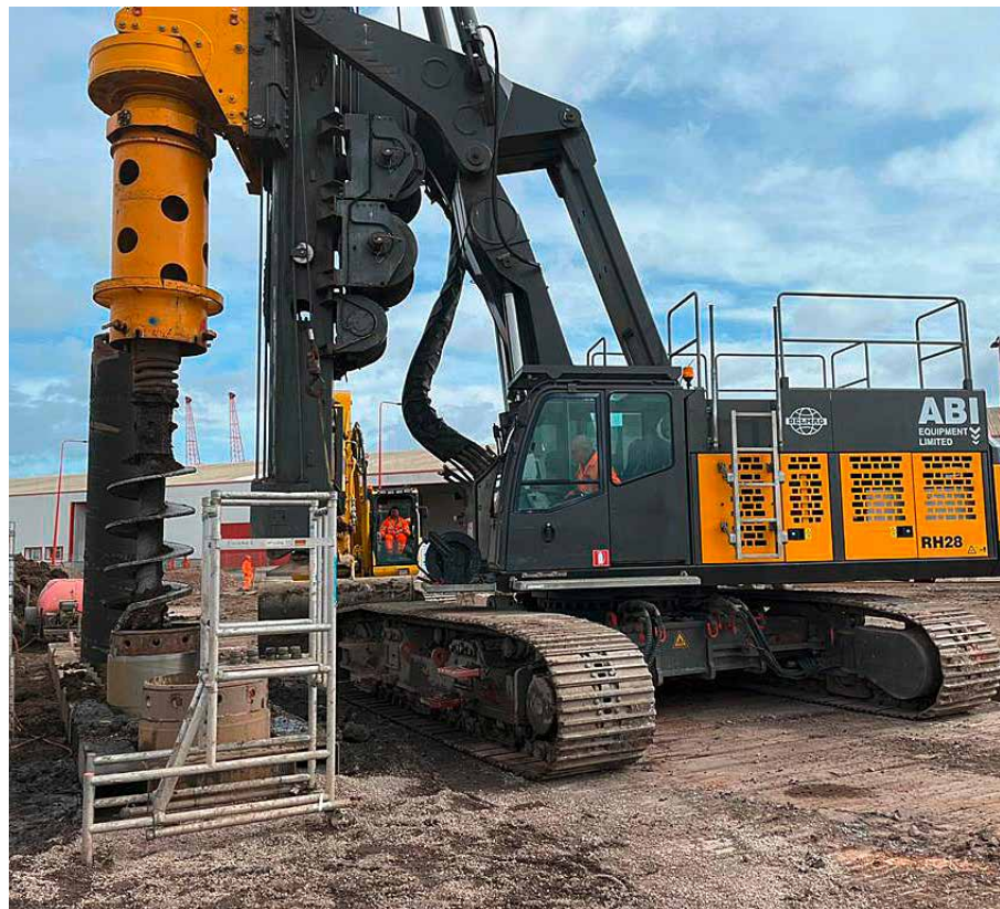
Photo: DELMAG drill rig RH 28 removing obstructions at the job site in Avonmouth
