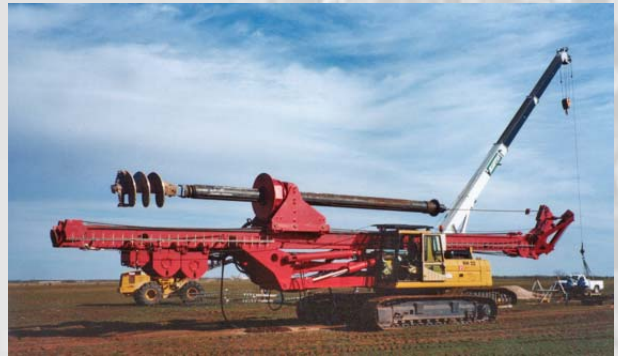
Drilling rig with folded down leader mast including rotary head, kelly bar and drilling tool for fast transfer on site
