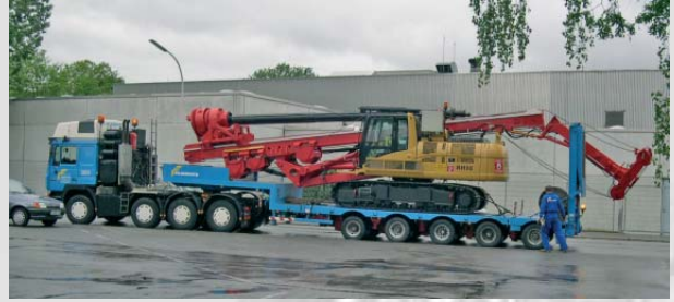
Transport of RH 10 with rotary head and kelly bar on the rig
