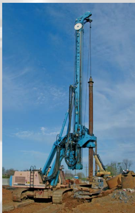
Drilling rig with short mast foot for drilling tools with large diameter
