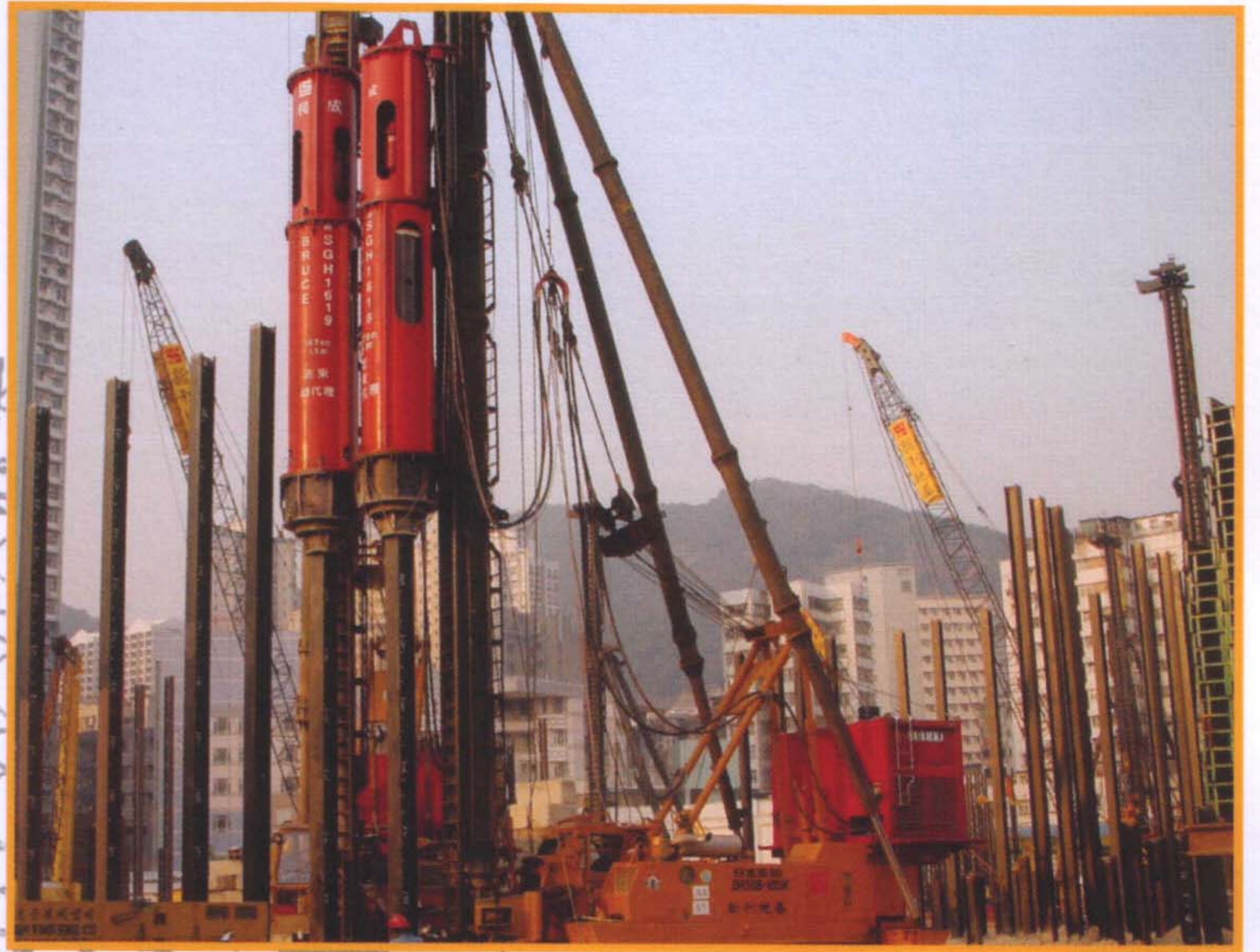
BRUCE SGH - 1618 & 1619 in Hong Kong driving H-beam piles (305 x 305, 223 kg/m, 12m length)
