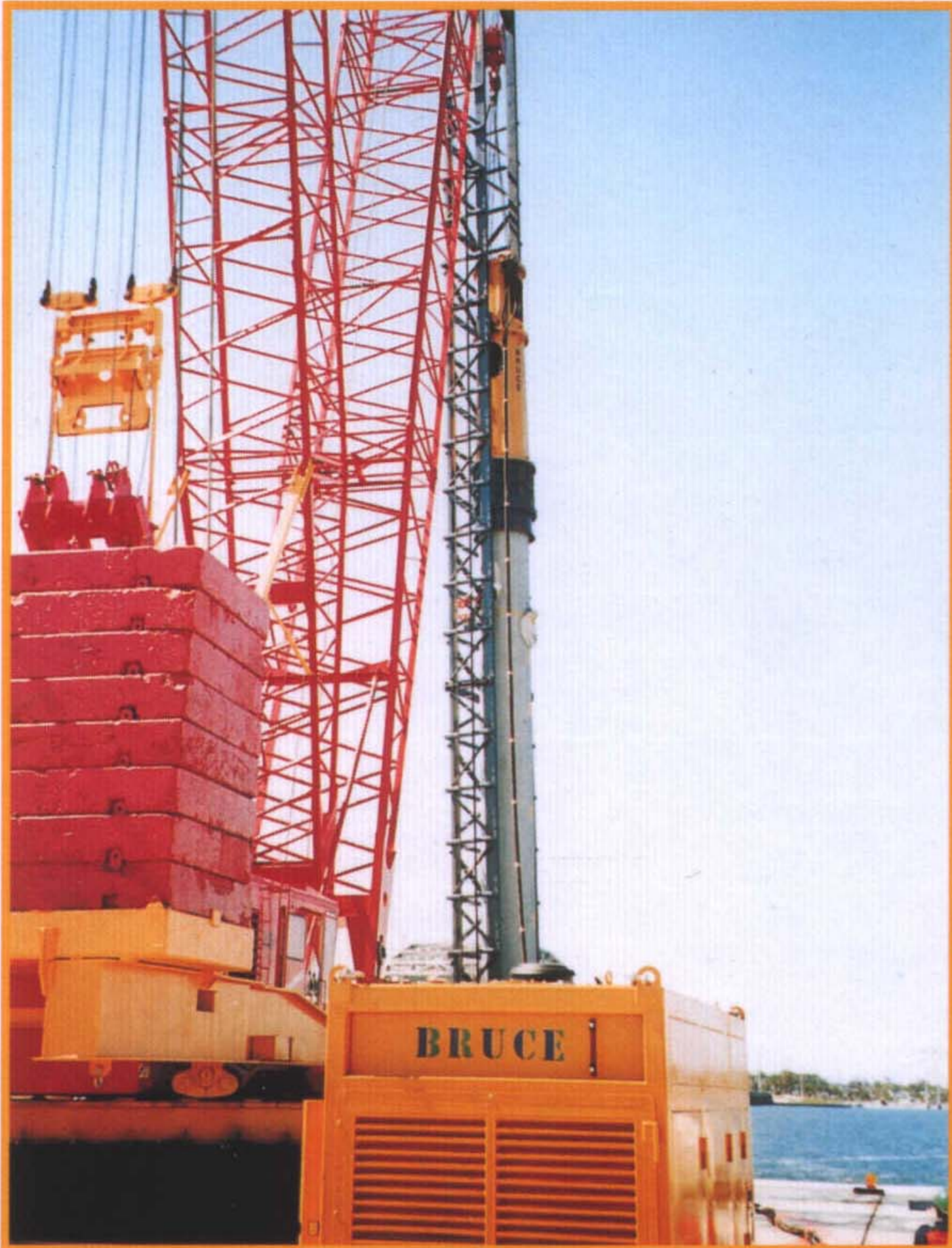
BRUCE SGH - 3013 working at bridge foundation site in Panama City, Florida driving concrete pile (O.D 60" x 1.D 45" x 120' length)
