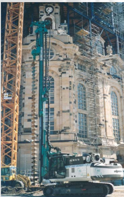
ABI MOBILRAM-System at work in front of the Frauenkirche in Dresden (Germany)
