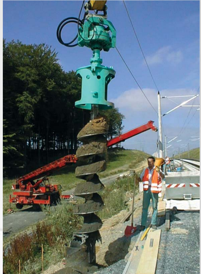
ABI auger drive with casing turn device for foundation piles along rail way
