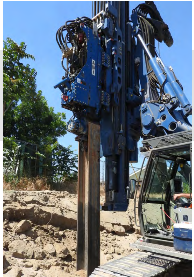
H-beam as a pile element are often used to improve the load bearing capacity of the ground.
