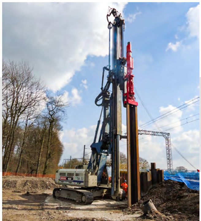
Driving steel sheet piles. DELMAG diesel pile hammer is often used for back driving or for embedding piles in a load bearing layer.
