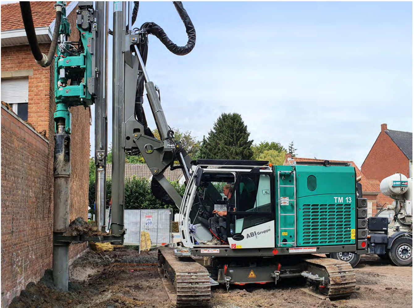
Installation of secant pile wall with a minimum distance to the existing structure using a VDW auger drive. The drilling and concreting is carried out in one continuous step, after drilling down concrete is pumped during withdrawal.
