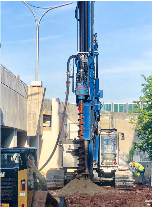
Installation of continuous flight auger piles: after reaching the desired depth during extraction concrete is pumped through the hollow stem of the auger.
