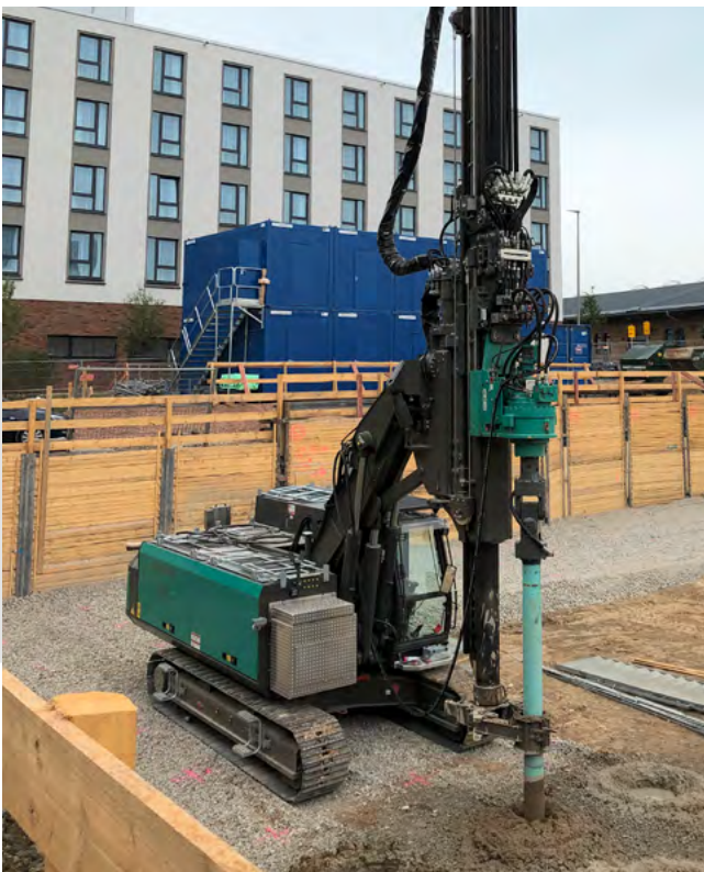
Increasing the load bearing capacity of the soil with mixed piles. Existing soil is mixed with aggregates while drilling and extracting.
