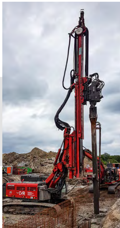
Displaceable soils are suitable for the installation of cast-in-situ full displacement piles.
