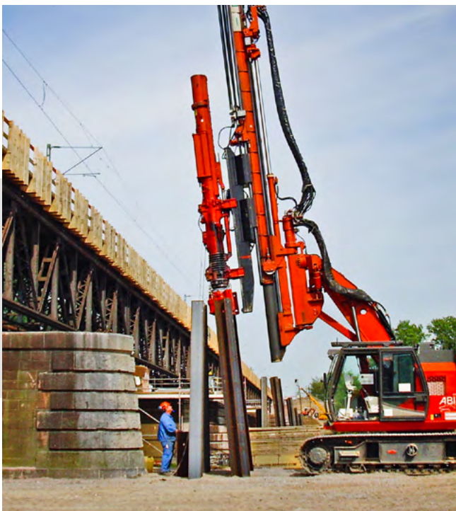
Impacting H-beams with DELMAG diesel pile hammer. With the DELMAG formula the load bearing capacity of the element can be calculated.
